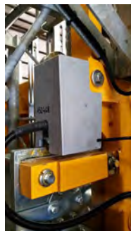
Example installation of a transducer
